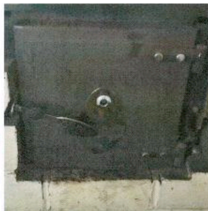
Door Air vent closed
